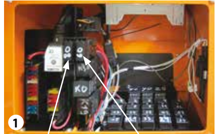
Preheating fuse Main fuse
