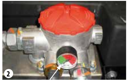
Clogging indicator on the hydraulic oil filter
