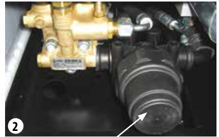
Water filter of the HP cleaner pump
